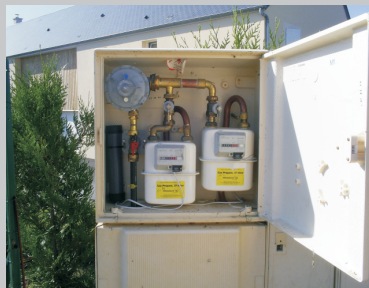
Figure 3 - Gas meter reading
