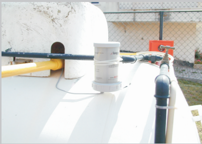
Figure 2 - LPG tank monitoring
